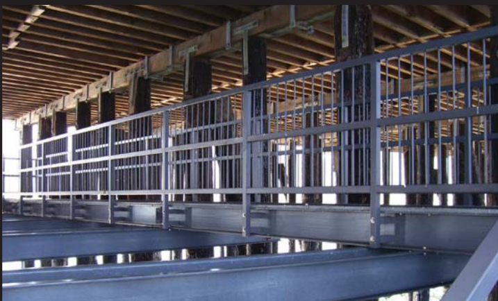
The Avila Beach Pier in California was reconstructed using EXTREN structural shapes for support, DURADEK® pultruded grating, stair treads and custom handrail.
