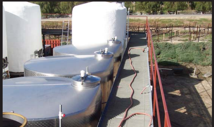
Strongwell's pultruded grating replaced rusted grating in a catwalk system for a California winery.
